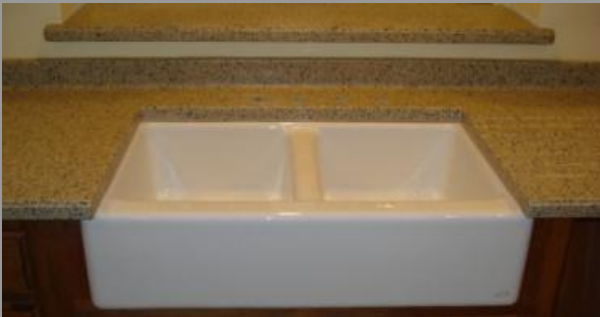
COUNTRY SINK INSTALLATIONS
